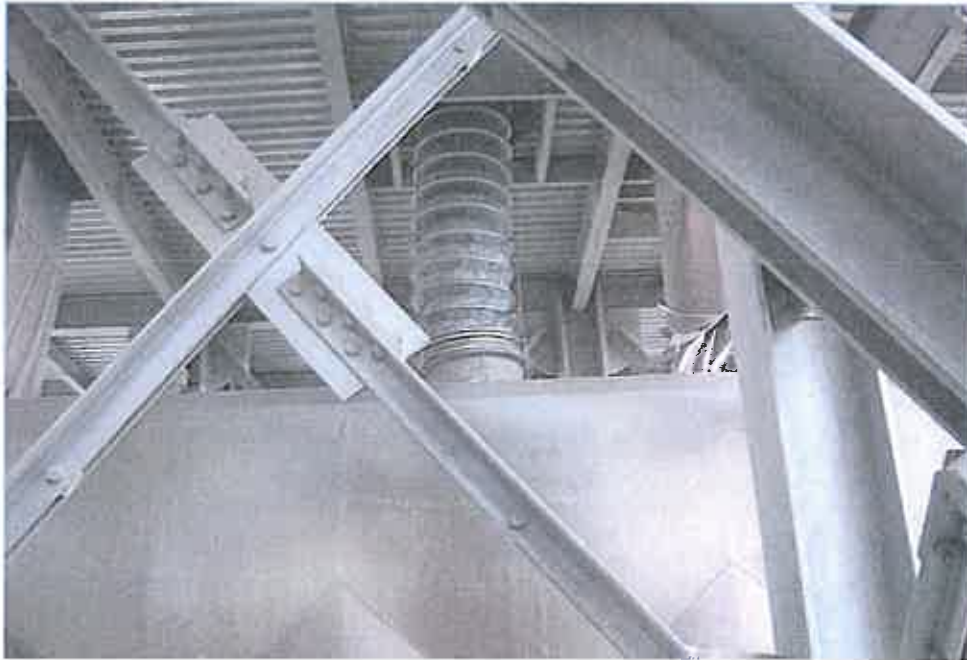
Figure 9 – Dry unloading chute for loading bulk trailers
